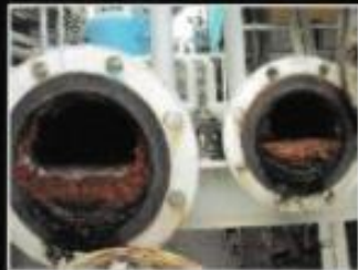
Rust, scale, fouling, ... in pipelines.
